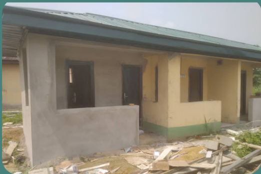
Before EMOC - Abandoned Classroom and Toilet, Idama Government Secondary School Project.
