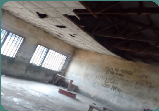
Before the EMOC Project: Alesa Comprehensive High School, Alesa, Eleme Local Government
