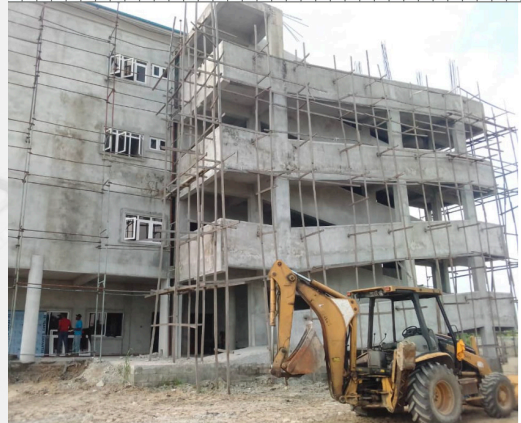
Ogba/Egbema/Ndoni: Omoku General Hospital Project in Progress. Contractor have returned to site
